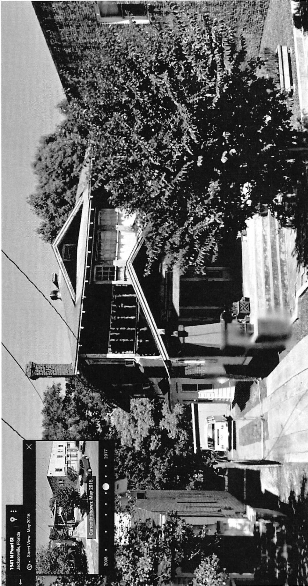
May 2015 Google Maps Photo indicating work continues with siding and window replacement
